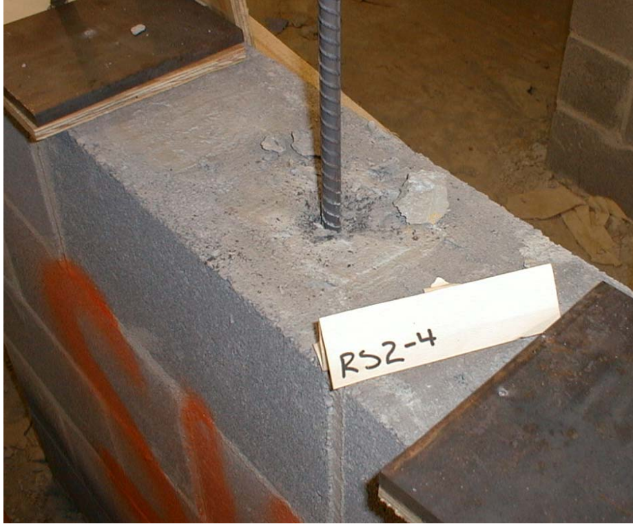
Figure 3. Typical small cone of grout that failed during testing of #4 bars
